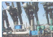
Loading / Offloading for trucks, railcars, ships
